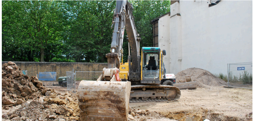
The team gets to work on building the new visitors' centre for families at HMP Wormwood Scrubs
